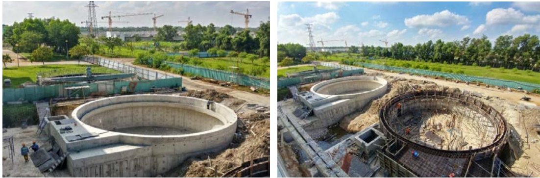
GRAVITY THICKENER TANK
